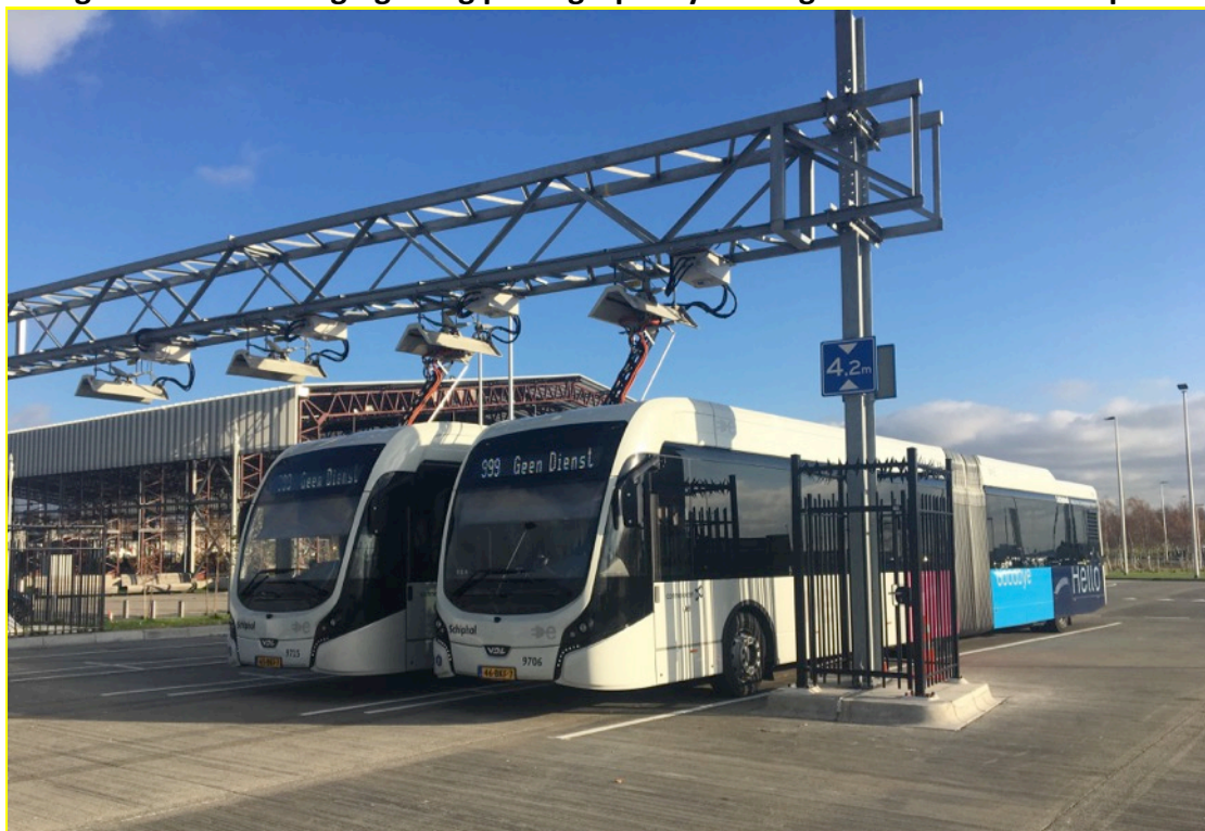
Figure 9: BEBs charging using pantograph style charger at Amsterdam Airport
